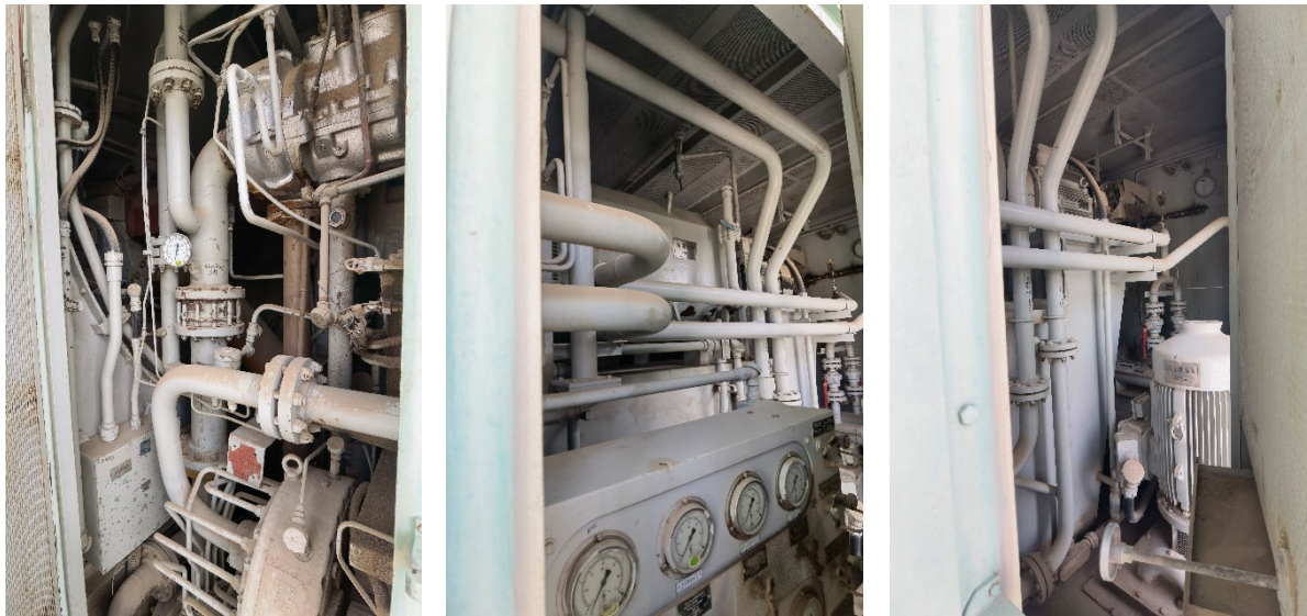
Liquid fuel system and lubricating oil system
