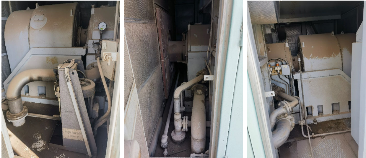
Bearing pedestal and jacking oil system of generator
