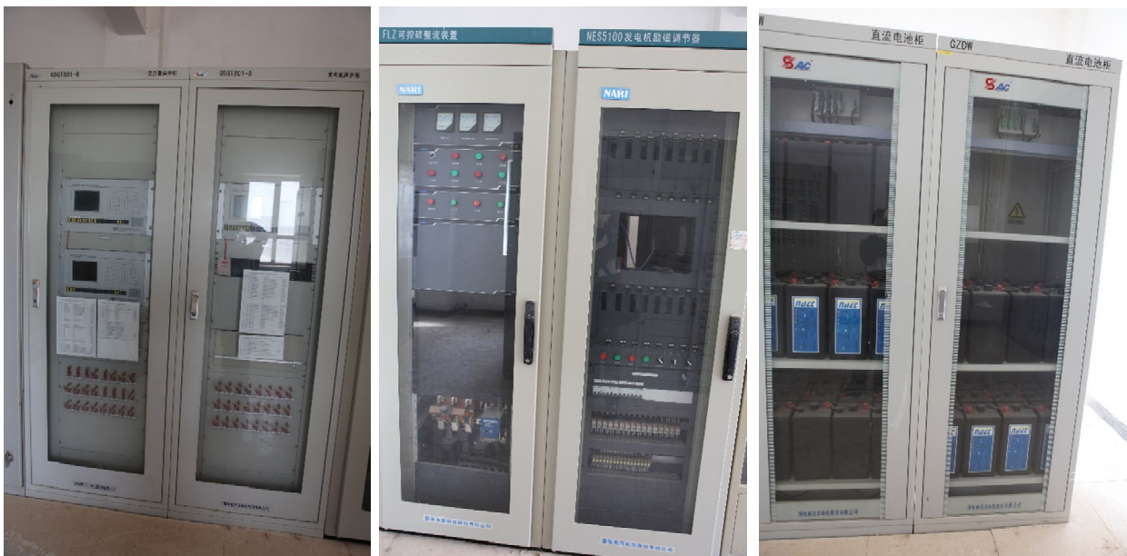
Transformer protection system, generator protection system, generator control system, DV power supply
