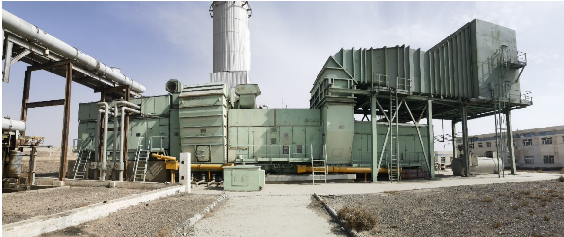
Panorama of power plant/电站全景图片
