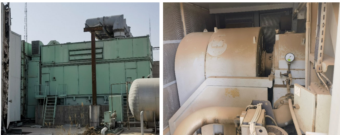
Generator and exciter
