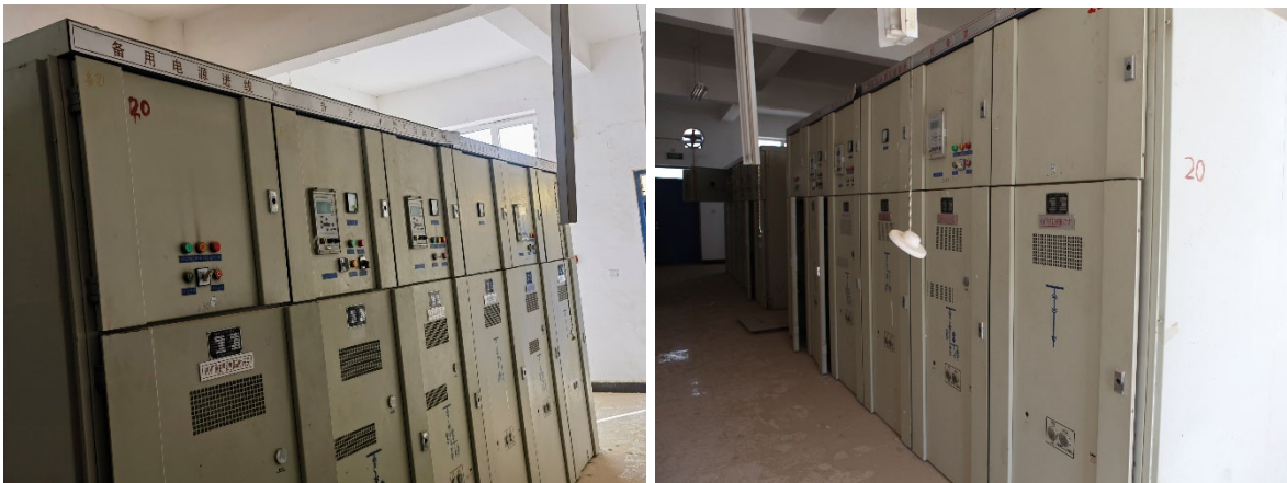
Electrical control cabinets
