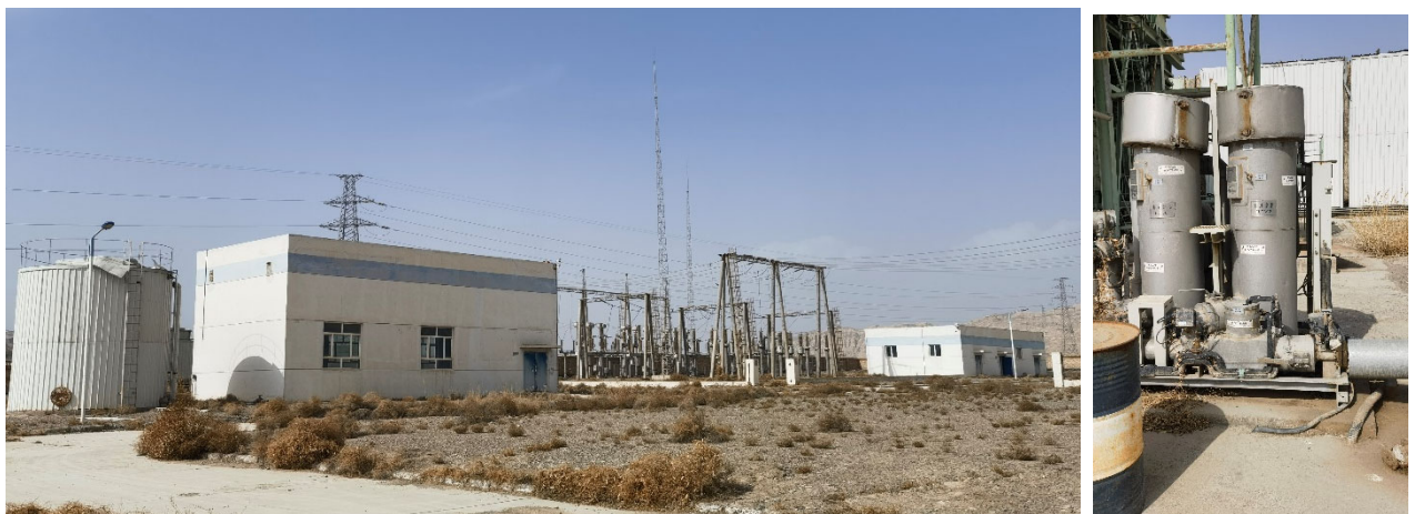
Power station transformer system and fuel oil system
